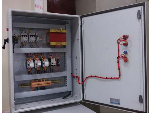
CONTROL PANEL WITH COMPLETE WIRING
