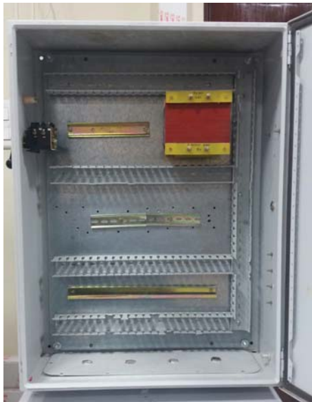
CONTROL PANEL WITH RACEWAYS/DIN RAILS
