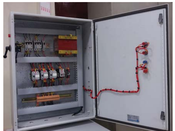
CONTROL PANEL WITH COMPLETE WIRING
