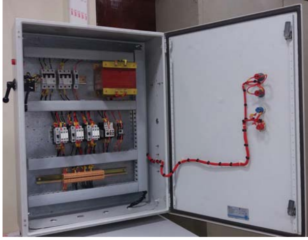
CONTROL PANEL WITH COMPLETE WIRING
