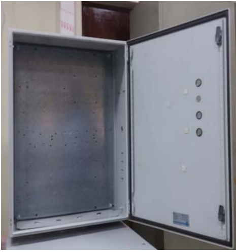
CONTROL PANEL WITH FIXING DRILL HOLES
