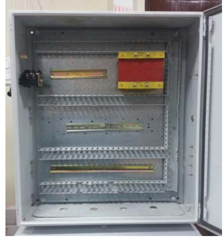
CONTROL PANEL WITH RACEWAYS/DIN RAILS
