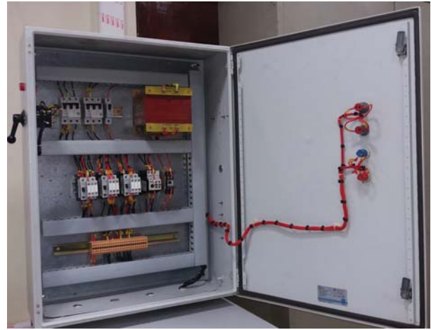
CONTROL PANEL WITH COMPLETE WIRING
