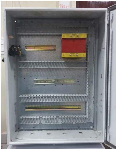
CONTROL PANEL WITH RACEWAYS/DIN RAILS
