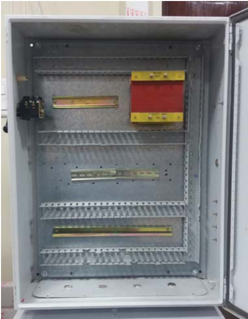
CONTROL PANEL WITH RAYS/DIN RAILS
