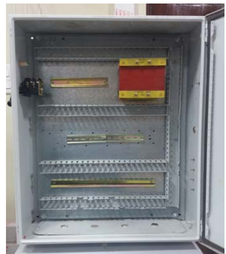
CONTROL PANEL WITH RACE WAYS/DIN RAILS
