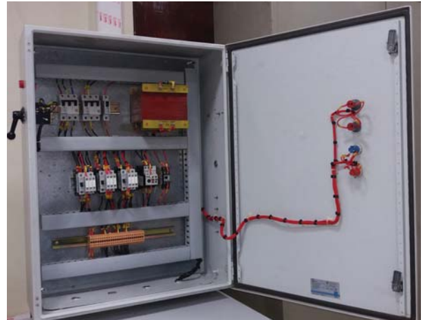
CONTROL PANEL WITH COMPLETE WIRING
