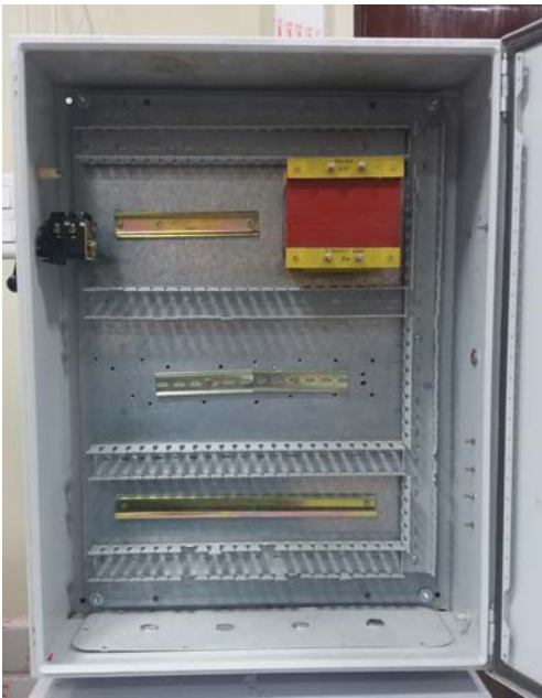
CONTROL PANEL WITH RAYS/DIN RAILS
