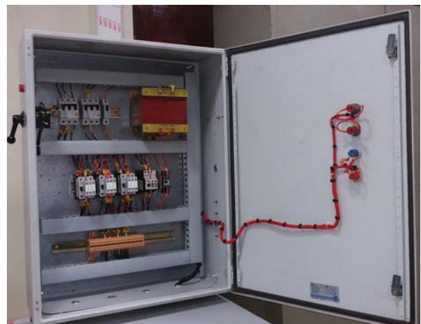
CONTROL PANEL WITH COMPLETE WIRING
