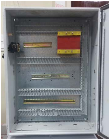
CONTROL PANEL WITH RACEWAYS/DIN RAILS
