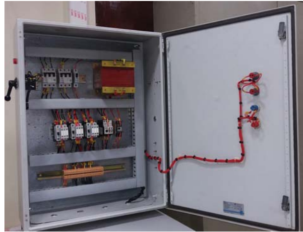
CONTROL PANEL WITH COMPLETE WIRING
