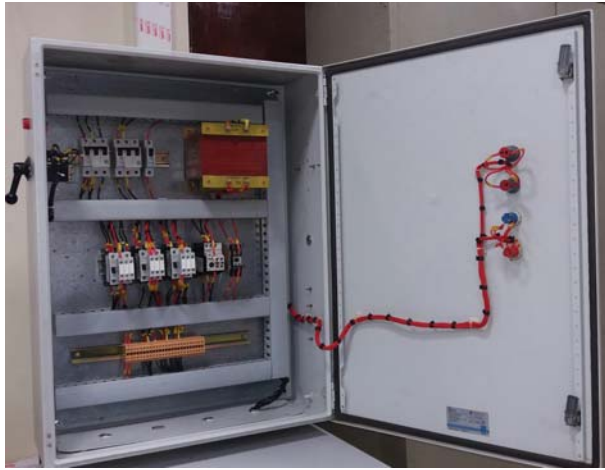
CONTROL PANEL WITH COMPLETE WIRING
