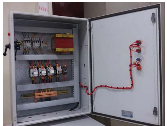
CONTROL PANEL WITH COMPLETE WIRING
