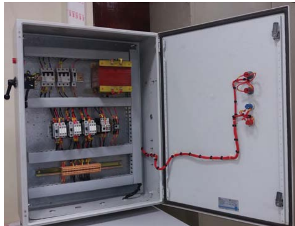
CONTROL PANEL WITH COMPELETE WIRING
