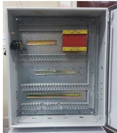
CONTROL PANEL WITH RACE WAYS/DIN RAILS
