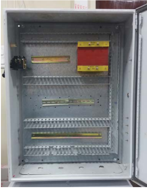
CONTROL PANEL WITH RACEWAYS/DIN RAILS
