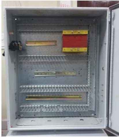
CONTROL PANEL WITH RACEWAYS/DIN RAILS
